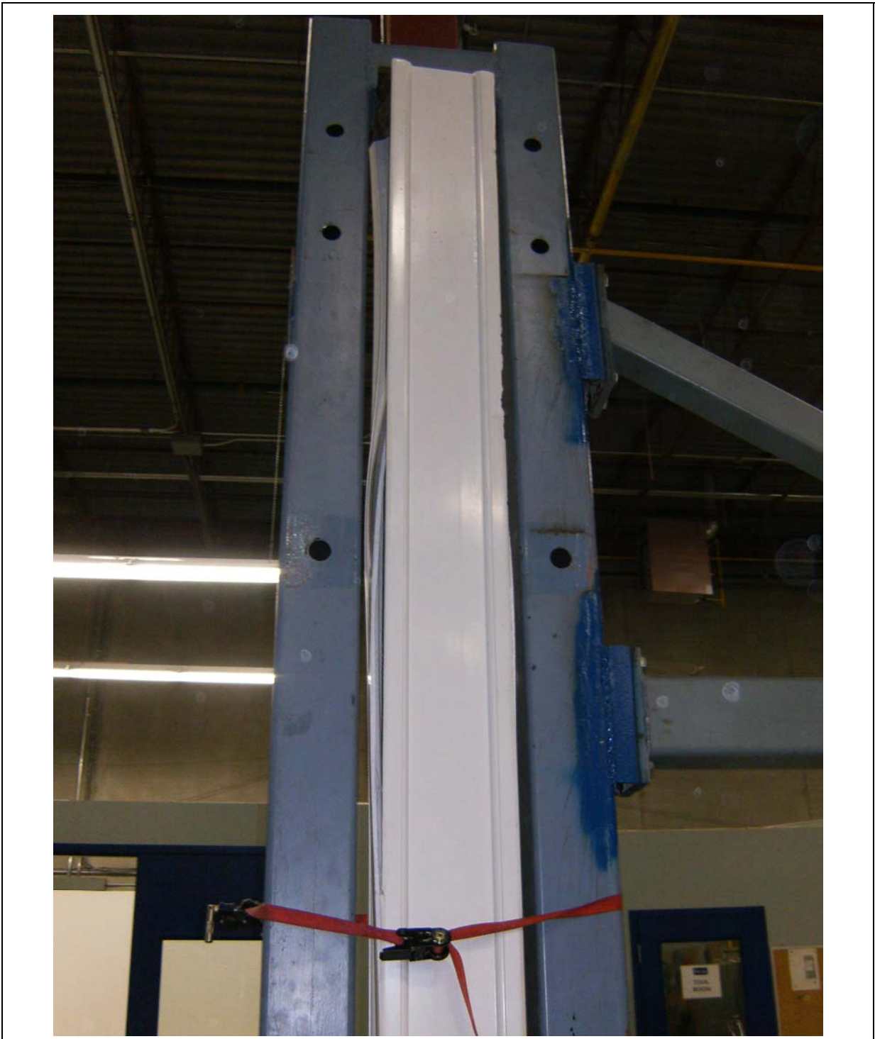
9-3/8 " Recessed Square Column Following Fracture
